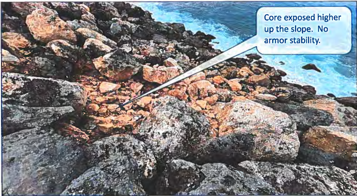
Photograph 3. Example of Exposed Core Aggregate
