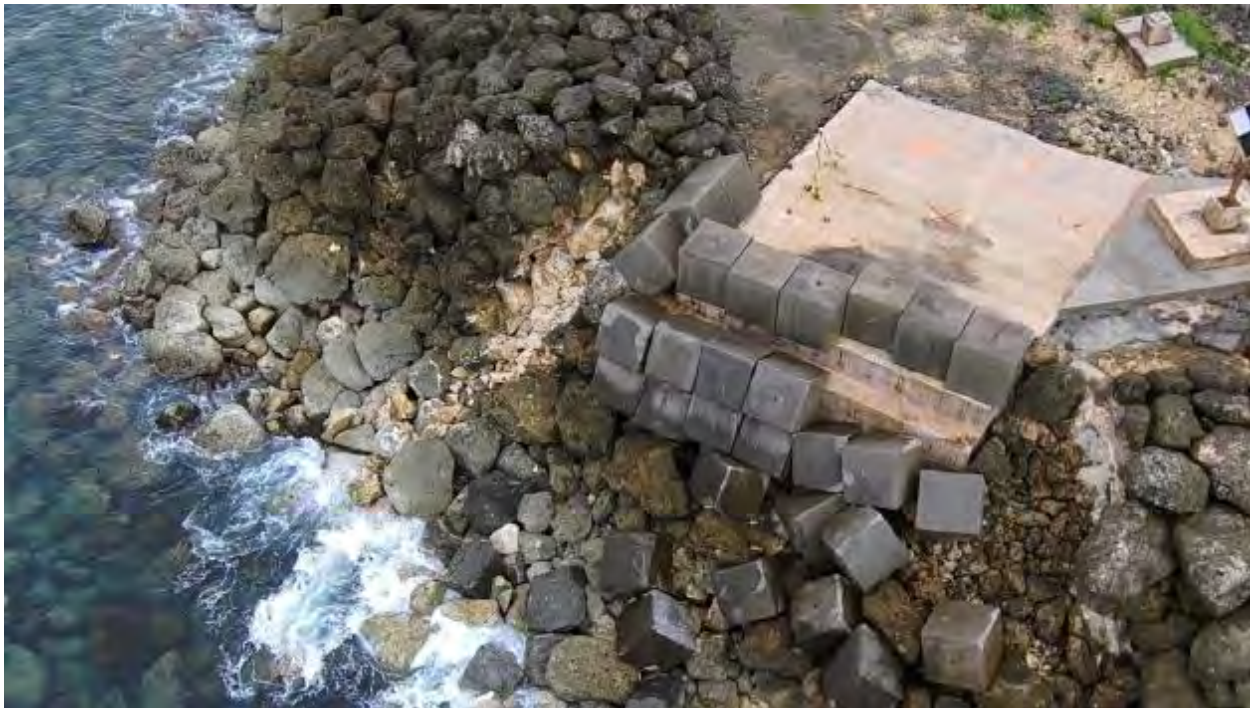
Figure 4. Large boulders and concrete blocks on a steep incline compose the Glass Breakwater armored shoreline.
